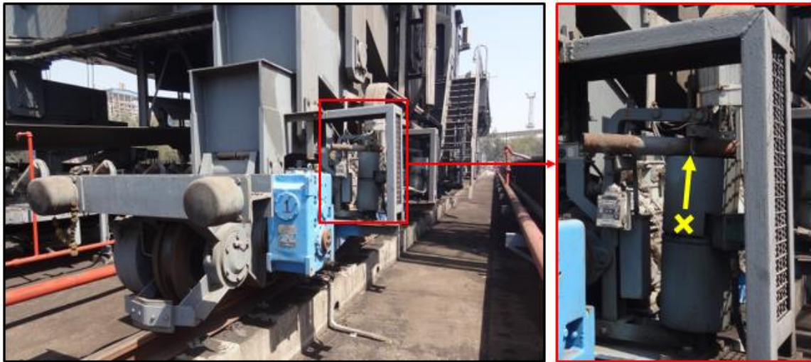
Brake Mechanically Blocked
