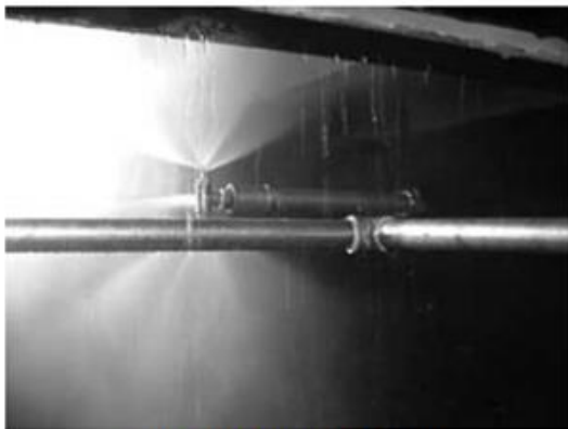
Fire-suppression System (A system to spray a combination of water and F-500)
